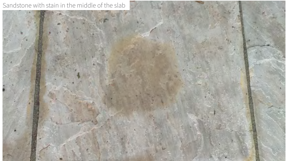
The same slab lifted up to show void directly underneath stain
