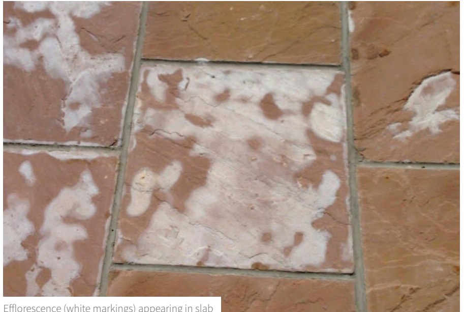
Efflorescence (white markings) appearing in slab
