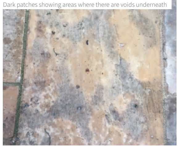
Dark patches showing areas where there are voids underneath
