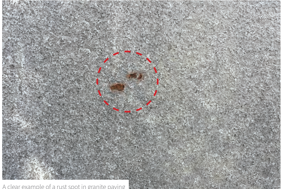
A clear example of a rust spot in granite paving
