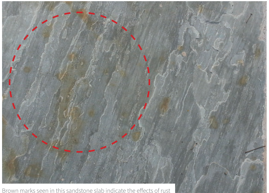
Brown marks seen in this sandstone slab indicate the effects of rust
